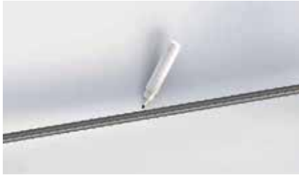
1. Mark the rebar with a marker pen half of coupler length from the end.
